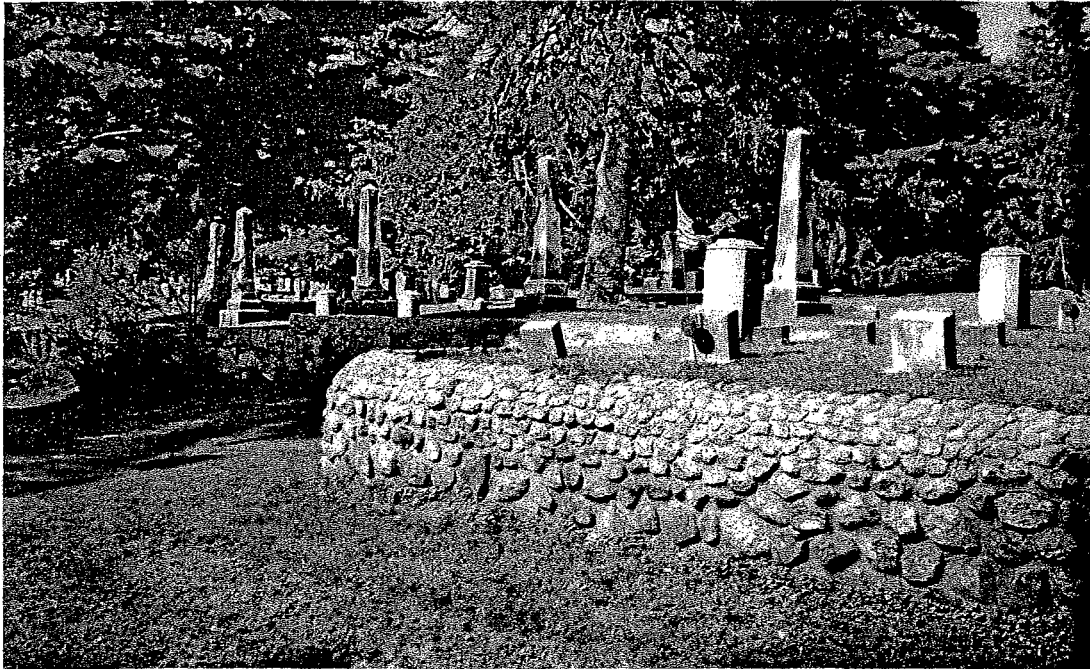
The Twitchell plot wall, a mortared rubble retaining structure, is in very good condition and can be improved through simple cleaning.
